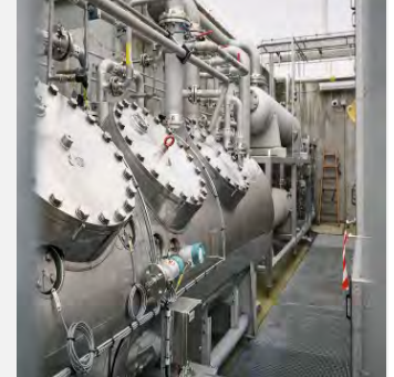
Ammonia catch system Max. 20ppm to atmosphere
