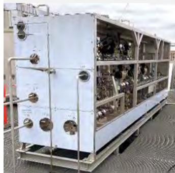
Fuel valve and return train (FVT)
