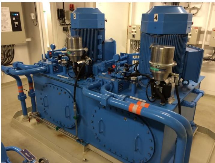
GreenOil filters installed on Steering Gear.
