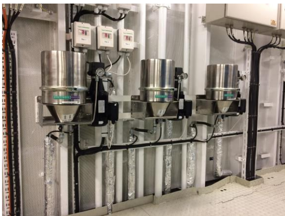
Three GreenOil filters are installed for each of the three Aux. Engines, which are into the operation instead of the purifiers.
