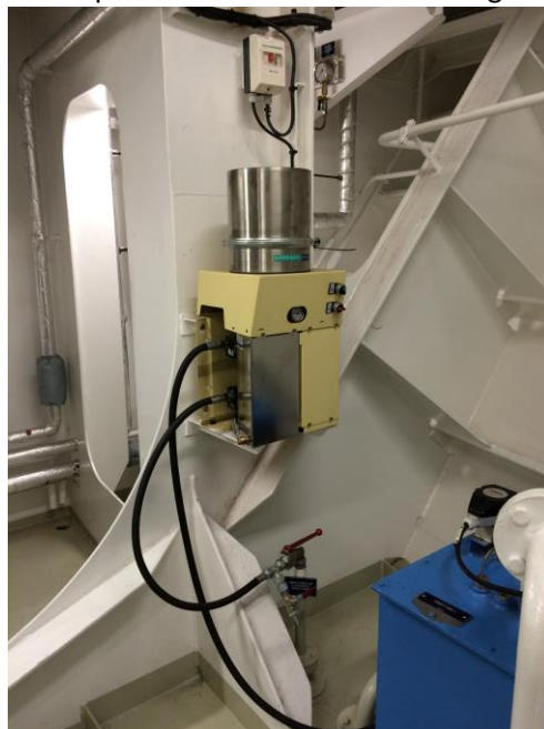
GreenOil filter installed on one of the Thrusters onboard Ark Germania.
